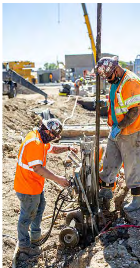
A new 66-inch wide pipe will bring wastewater into the Plant. Workers fill gaps around the pipe with soil after removing 40-foot-long sheet piles installed to help bury the pipe underground.
