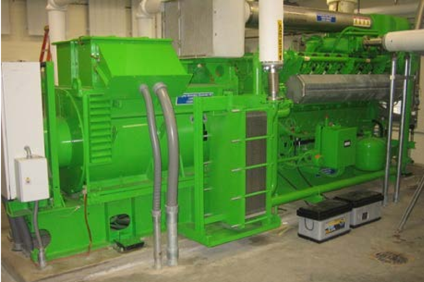
Figure 15 IC ENGINE ELECTRICAL & COMBINED HEAT AND POWER PLAN MASTER PLAN AND PRIMARY TREATMENT DESIGN CITY OF SUNNYVALE
