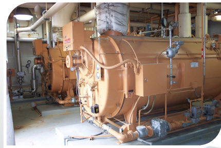
Dual Fuel Boiler
