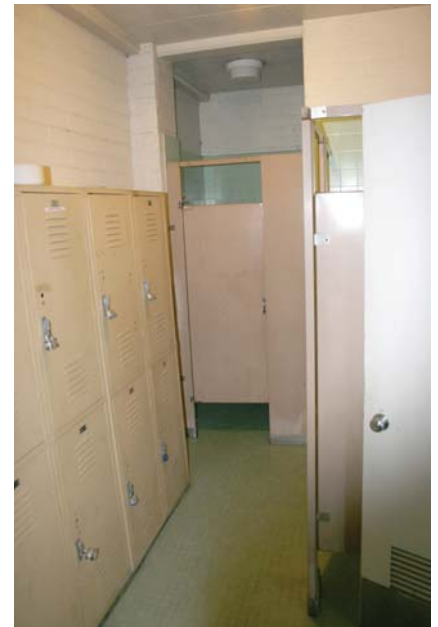
Staff Restrooms - Do not meet accessibility codes
