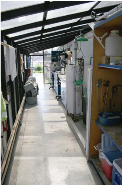
Compliance Inspection Lab - Unconditioned 'porch' space and insufficient storage area
