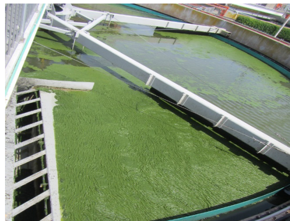
Figure 6: Fixed Growth Reactor (top) distributing wastewater over plastic growth media. Dissolved Air Flotation Tank (bottom) processing secondary solids
