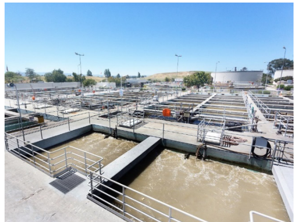
Figure 4: Preliminary and primary treatment processes. Barrel grinders (top), and Preaeration Basins and Primary Sedimentation Tanks (bottom)
