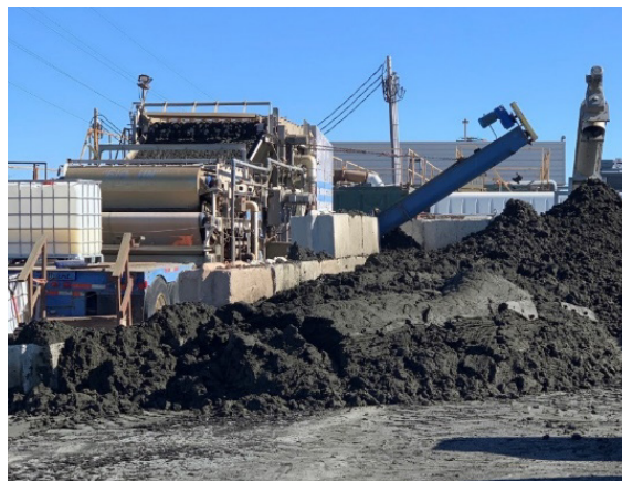
Figure 9: Biosolids dewatering operation
