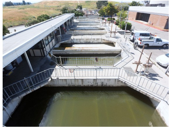
Figure 7: Dual Media Filters treating wastewater
