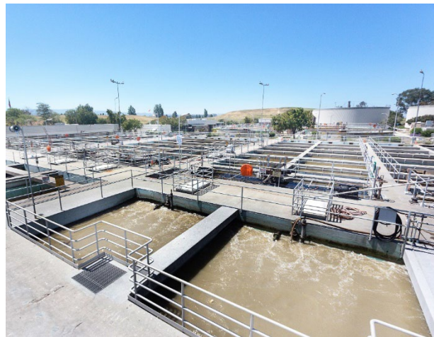
Figure 5: Barrel grinders (top), and Preaeration Basins and Primary Sedimentation Tanks (bottom)
