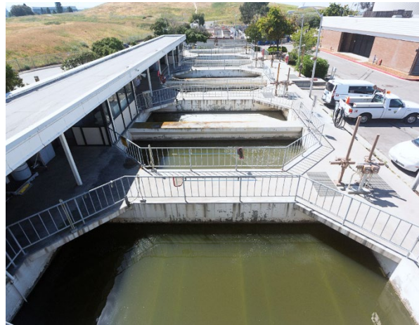
Figure 9: Dual Media Filters treating wastewater
