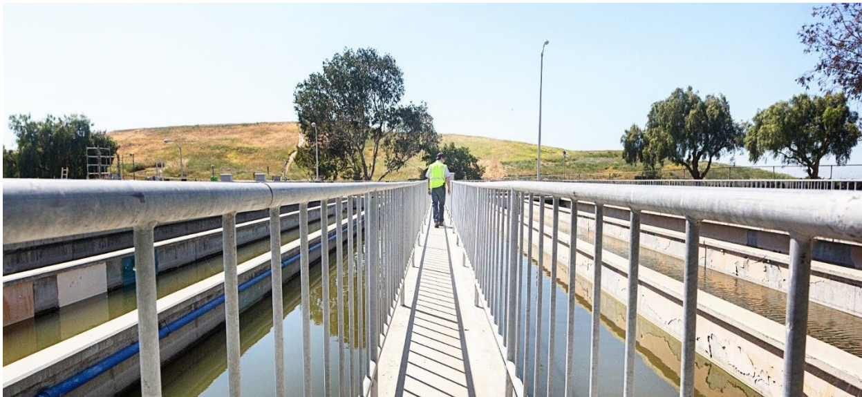
Figure 10: Wastewater being disinfected in the Chlorine Contact Tanks prior to discharge into Moffett Channel
