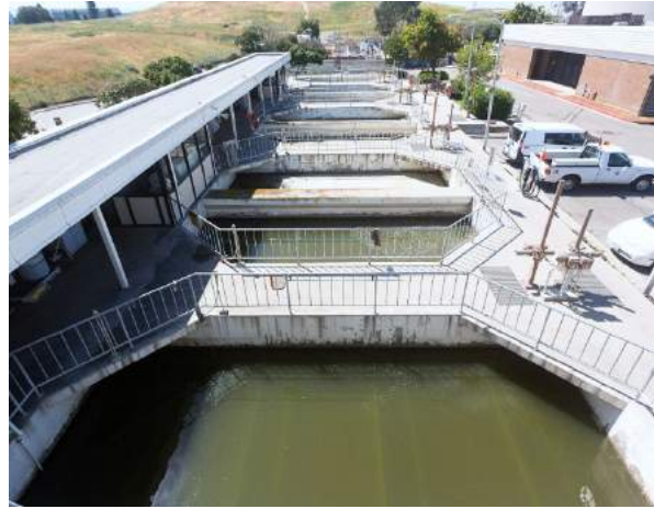
Figure 9: Dual Media Filters treating wastewater
