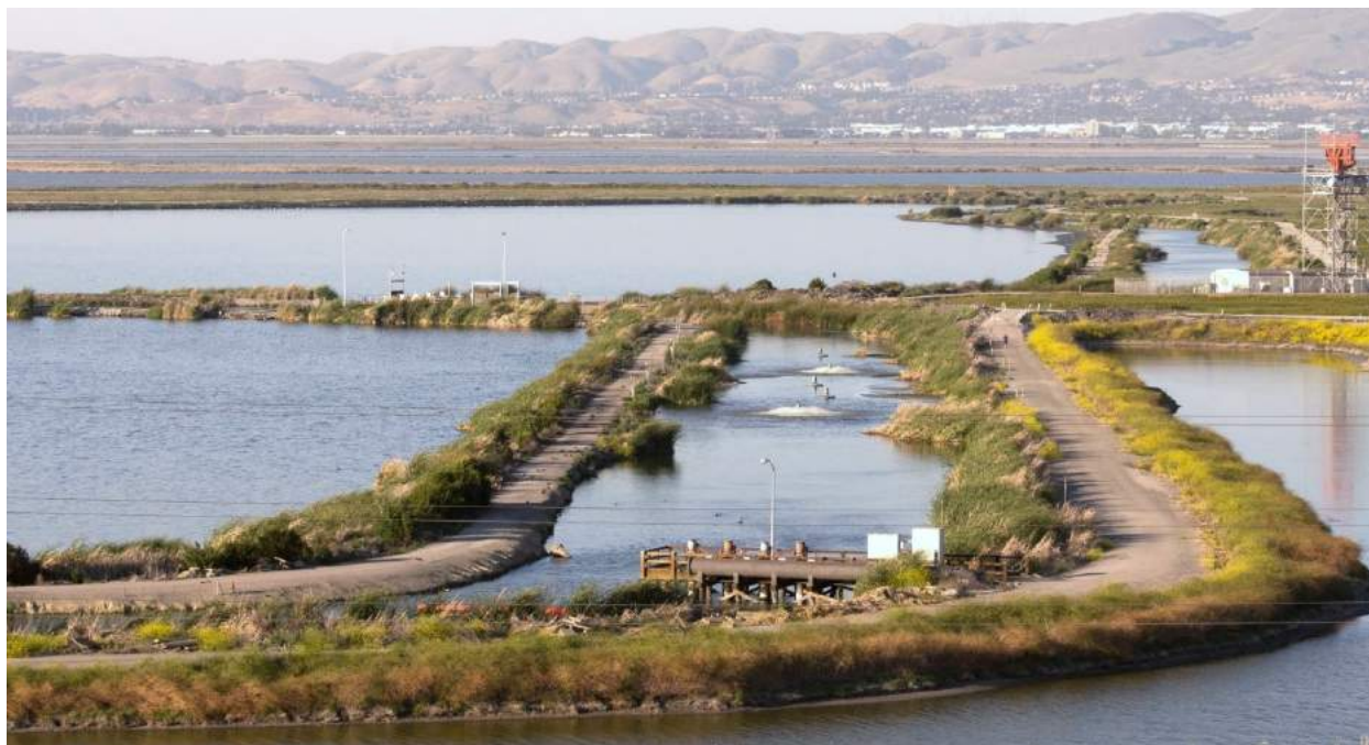
Figure 6: Oxidation Ponds, including the return/distribution channel, Pond Effluent Pump Station, and surface aerators
