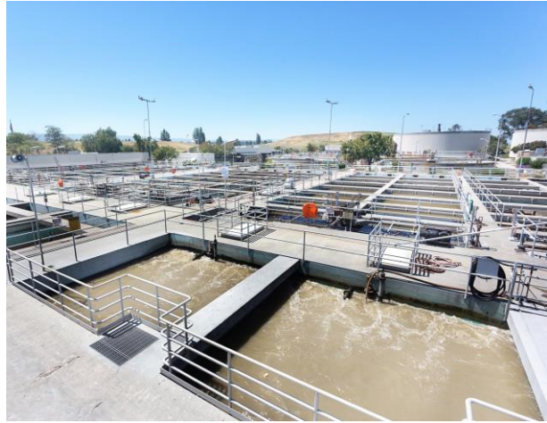
Figure 5: Preaeration Tanks and Primary Sedimentation Basins
