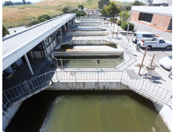
Figure 9: Dual Media Filters treating wastewater
