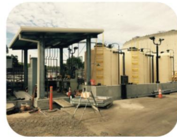
New Sodium Hypochlorite Tank Farm
