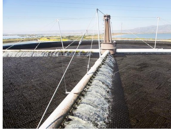
Figure 8: Fixed Growth Reactor distributing wastewater over plastic growth media
