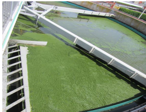
Figure 7: Algae being skimmed off the surface of wastewater in a Dissolved Air Flotation Tank
