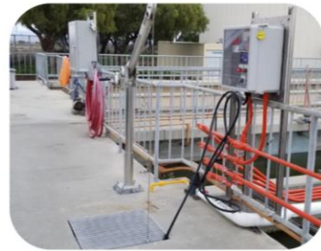
New Sodium Bisulfite (SBS) Dosing Point
