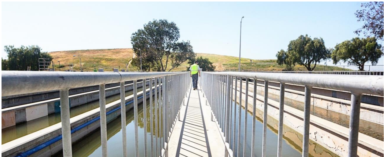
Figure 10: Wastewater being disinfected in the Chlorine Contact Tanks prior to discharge into Moffett Channel
