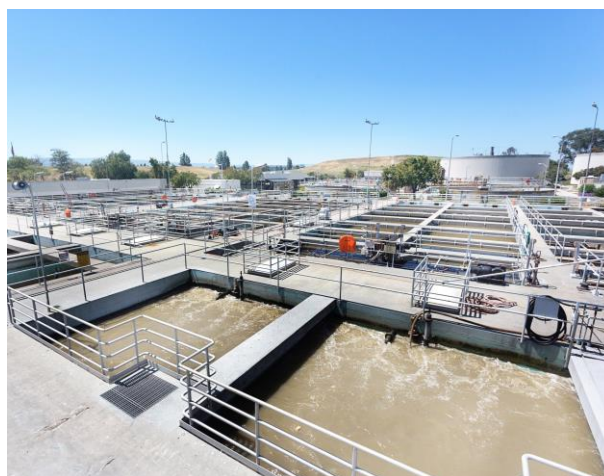
Figure 5: Preaeration Tanks and Primary Sedimentation Basins
