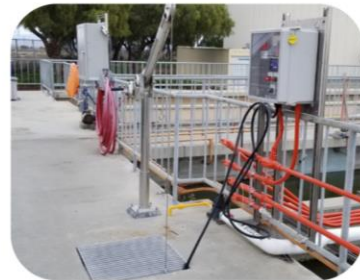
New Sodium Bisulfite (SBS) Dosing Point
