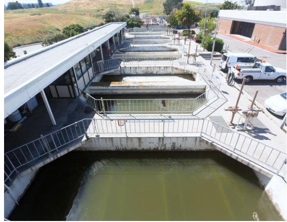
Figure 9: Dual Media Filters treating wastewater
