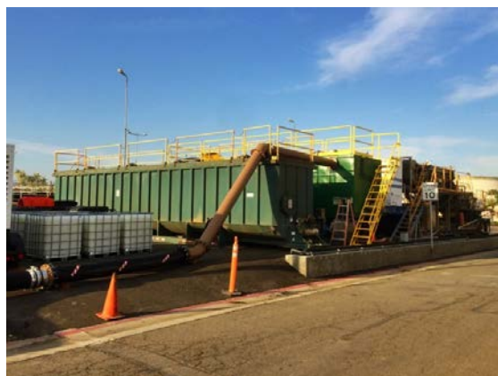
Figure 11: Solids dewatering operation
