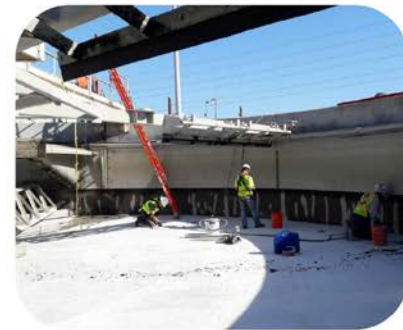
Contractor assessing an Air Floatation Tank
