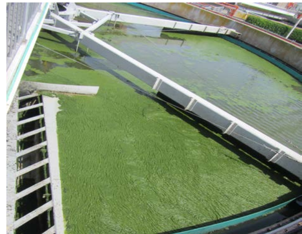
Figure 8: Algae being skimmed off the surface of wastewater in a Dissolved Air Flotation Tank
