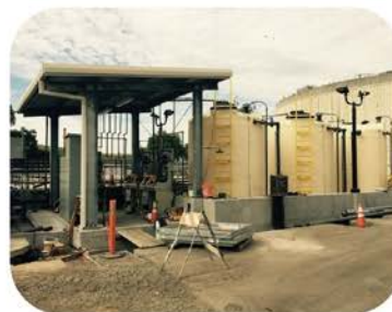
New sodium hypochlorite tank farm
