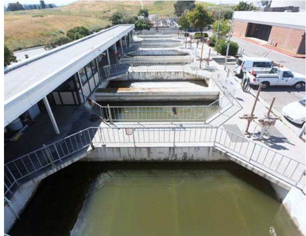
Figure 9: Dual Media Filters treating wastewater
