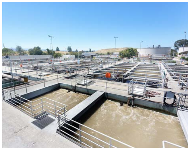
Figure 5: Preaeration Tanks and Primary Sedimentation Basins
