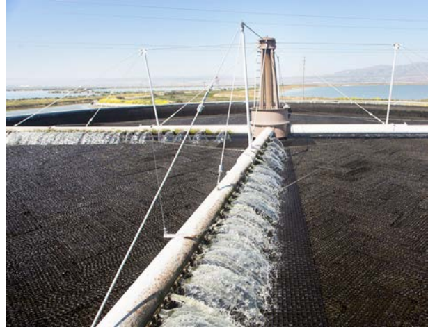
Figure 7: Fixed Growth Reactor distributing wastewater over plastic growth media
