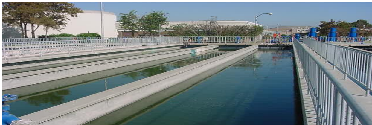
Figure 10: Wastewater being disinfected in the Chlorine Contact Tanks prior to discharge into Moffett Channel
