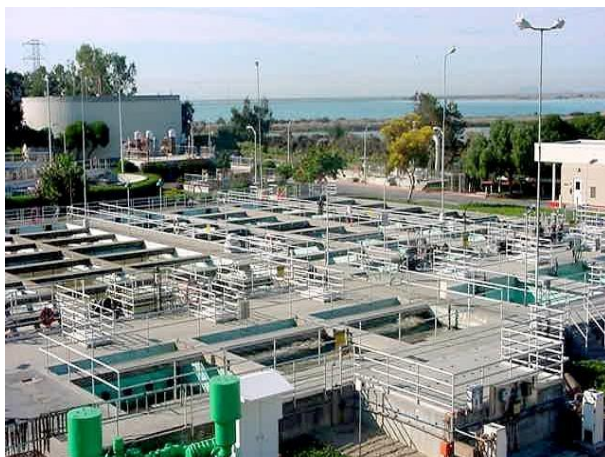
Figure 5: Preaeration Tanks and Primary Sedimentation Basins
