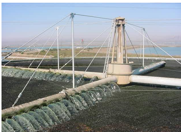
Figure 7: Fixed Growth Reactor distributing wastewater over plastic growth media
