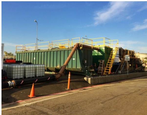
Figure 11: Solids dewatering operation
