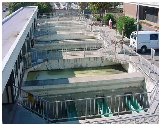
Figure 9: Dual Media Filters treating wastewater
