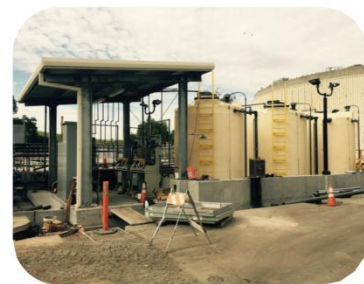
New sodium hypochlorite tank farm
