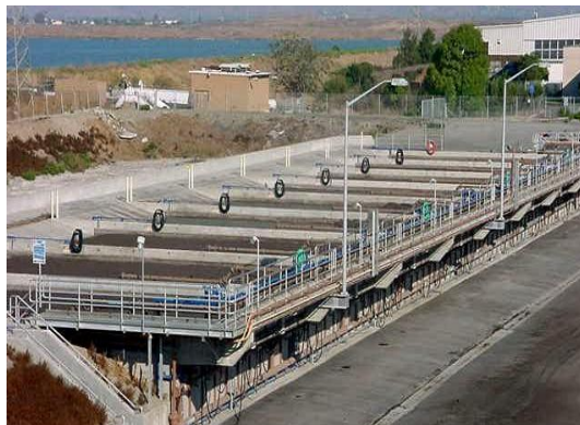
Figure 12: Dewatering Beds treating biosolids
