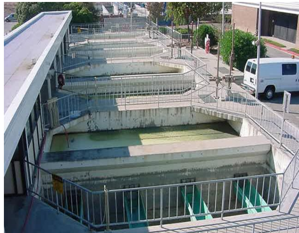
Figure 9: Dual Media Filters treating wastewater
