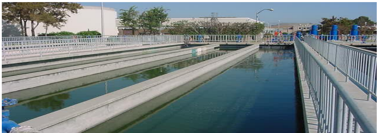
Figure 10: Wastewater being disinfected in the Chlorine Contact Channels prior to discharge into Moffett Channel
