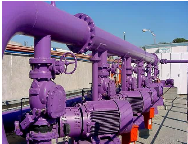
Figure 14: WPCP Recycled Water distribution piping
