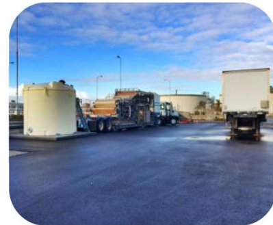
New Synagro Dewatering Area
