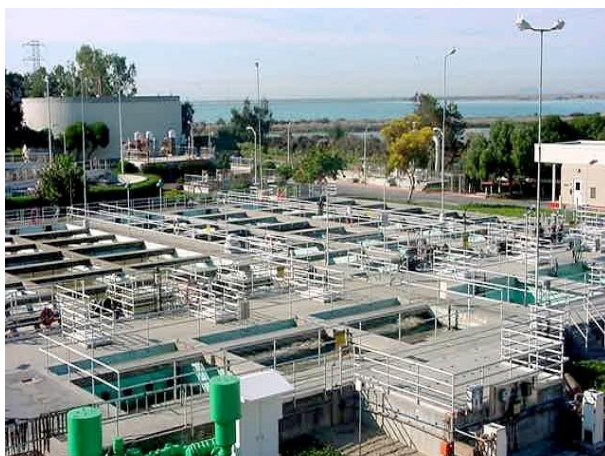
Figure 5: Preaeration Tanks and Primary Sedimentation Basins
