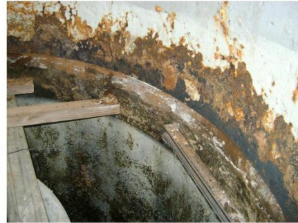
This photo, taken in 2009, gives us a glimpse inside one of the aging AFTs.
