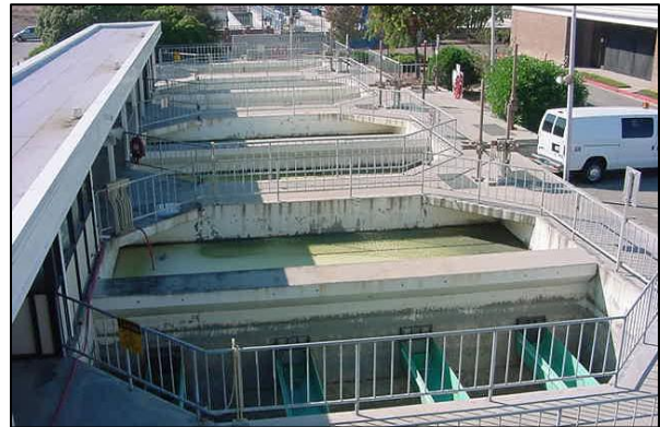
Figure 8: DMFs Treating FGR Effluent
