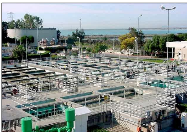
Figure 4: Preaeration Tanks and Primary Sedimentation Basins
