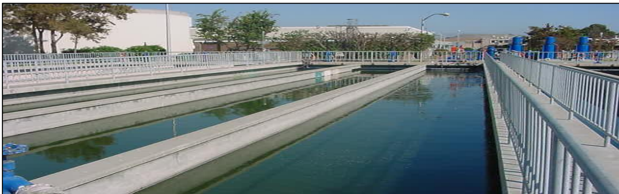
Figure 9: Chlorine Contact Channels Treating DMF Effluent Prior to Discharge to Moffett Channel
