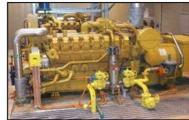
Figure 11: One of Two Caterpillar Power-Generating 1130 HP Reciprocating Internal Combustion Engines
